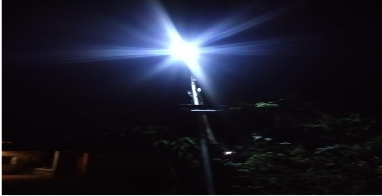
Solar Lights After installations
